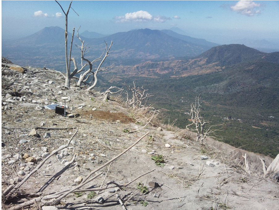
Figure 8. VSMG station, installed on the upper northern flank of the volcano, made by a reinforced concrete cube buried in the pyroclastic material, where the self-centering benchmark was anchored.
