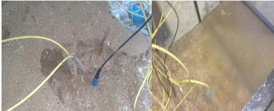
Figure 8. Failure at the toe of the slope and runoff at the toe (dense slope).
