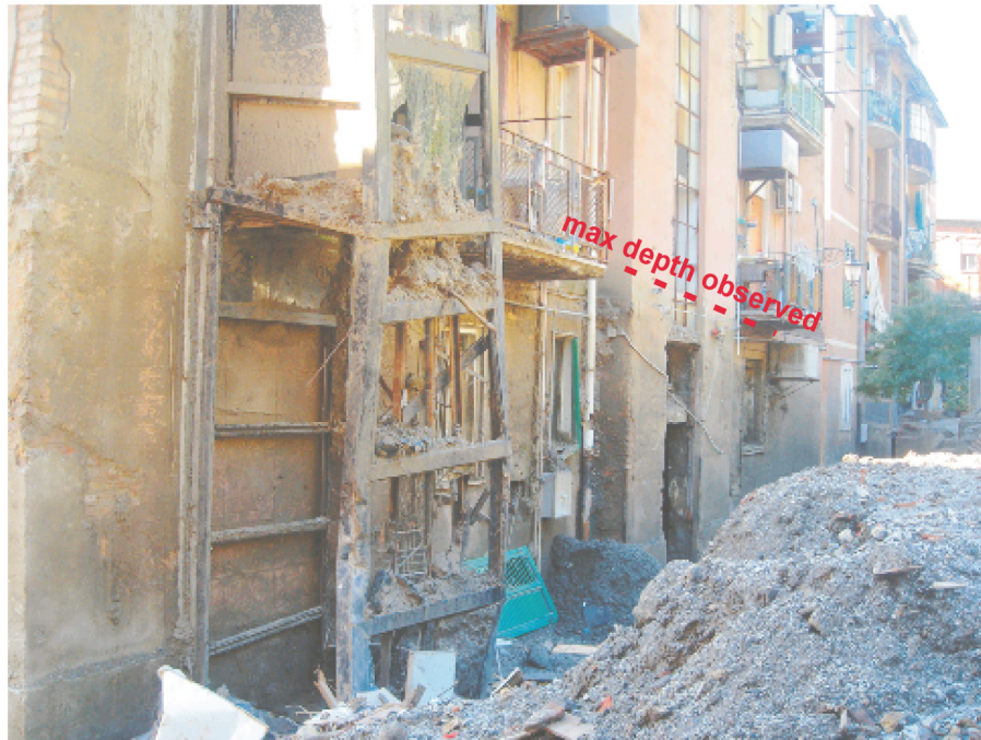
Figure 5. Evidences on the wall of the maximum depth observed during the event.
