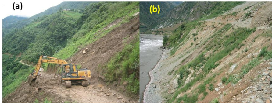
Figure 7. (a) A section of the FG2 road several kilometers north of Fugong that was temporarily closed by a landslide; and (b) secondary road to a small mountain village near Daxingdi (not included in our landslide survey) that was abandoned during construction because of excessive landslides.
