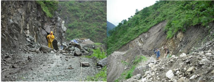
Figure 2. The highest landslide erosion occurred along a 1 yr old road (DXD) leading to a remote village and a future hydropower plant just south of Daxingdi, Yunnan, China.
