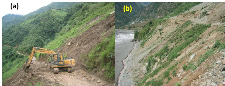
Figure 7. (a) A section of the FG2 road several kilometers north of Fugong that was temporarily closed by a landslide; and (b) secondary road to a small mountain village near Daxingdi (not included in our landslide survey) that was abandoned during construction because of excessive landslides.
