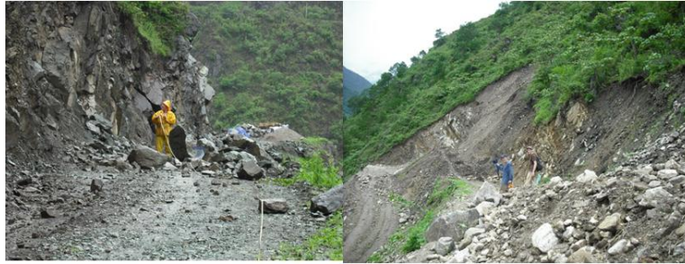
Figure 2. The highest landslide erosion occurred along a 1 yr old road (DXD) leading to a remote village and a future hydropower plant just south of Daxingdi, Yunnan, China.
