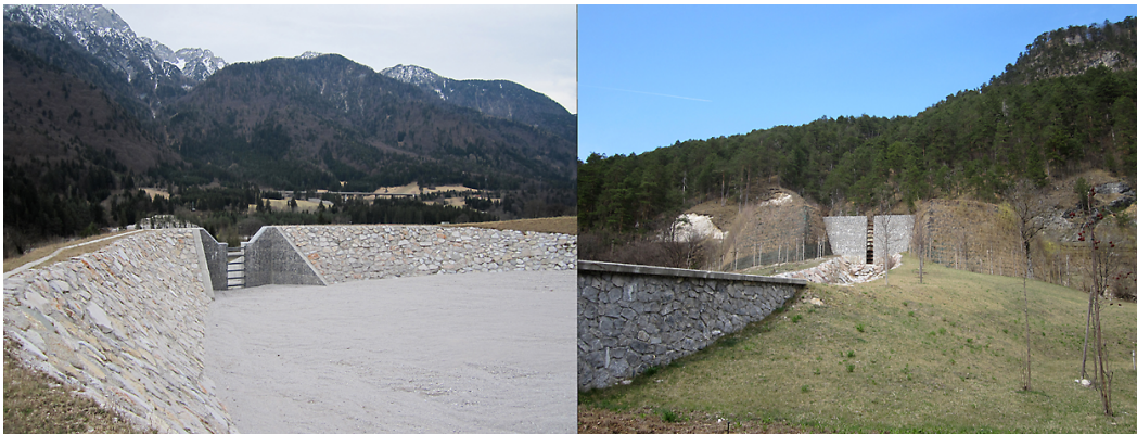
Fig. 6. Structural debris flow mitigation measures in Malborghetto-Valbruna, Italy.
