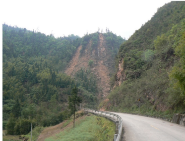
(b) Shallow slope failures (by Dr. M.M. Wang)
