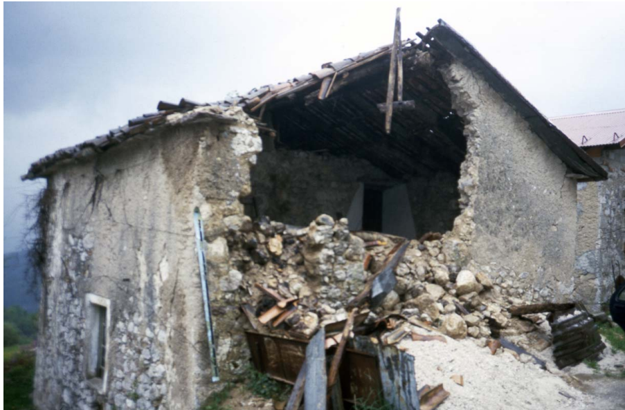
Fig. 7. Damage to buildings in Drežniške Ravne after the 1998 earthquake (photo: Matija Zorn).
