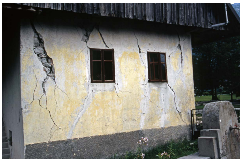
Fig. 8. Damage to buildings in Čezsoča after the 2004 earthquake (photo: Matija Zorn).
