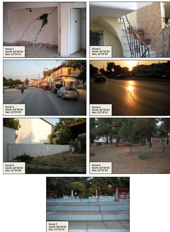
Fig. 11. Field evidences of ground ruptures in Perea. Coordinates are in UTM WGS 84 (projected). Damages witnessed at buildings (points 1 and 2), streets pavement (points 3 and 4), light constructions (points 5 and 7) and natural terrain (point 6).
