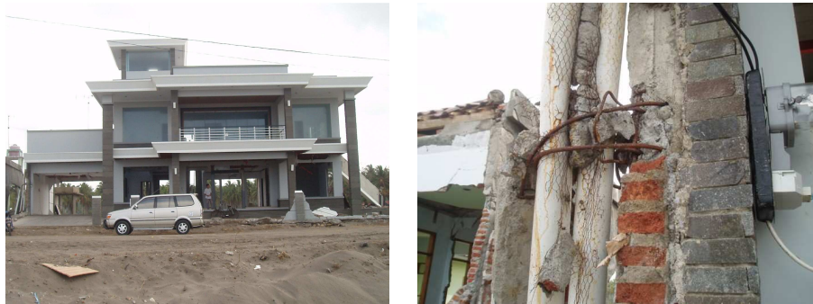
Fig. 14. Well engineered beachfront villa after inundation to a depth of 3.8 m (a). Reinforcement detail is shown at right (b).
