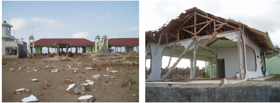
Fig. 13. Two relatively well-made apartment complexes (a) with rudimentary reinforced concrete columns (b), after inundation to a depth of 3.8 m.
