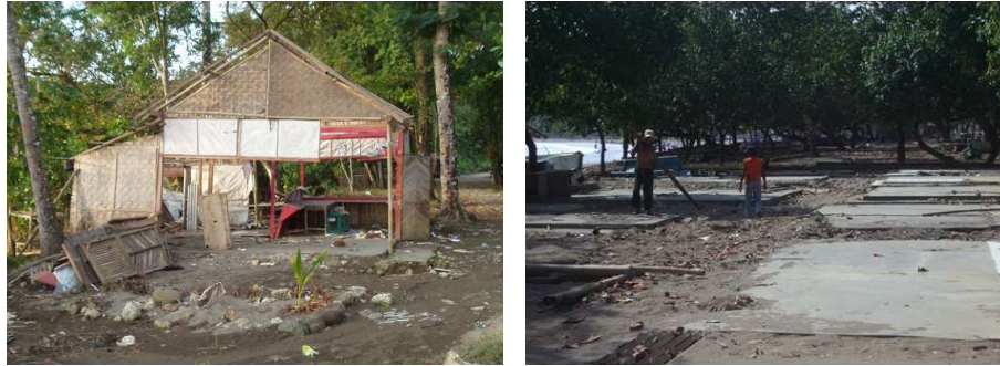
Fig. 11. Typical damage to semi-permanent wooden shops, after inundation to nearly 1 m depth (a) and to 3 m (b). Only the concrete floors remain in the right image, where prior to the tsunami there had been a row of more than 30 shops.
