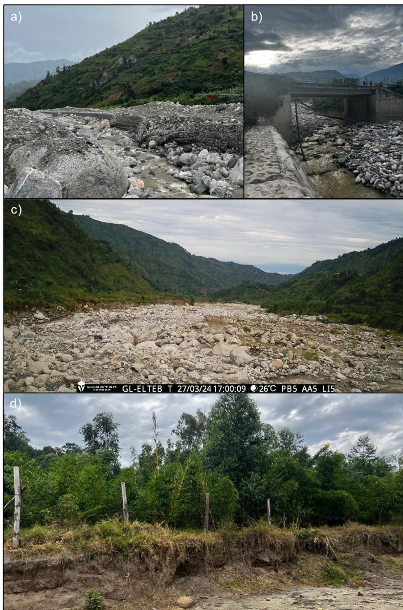
Figure M1. Photographs taken during June 2023 field reconnaissance: (a) collapsed gabions adjacent to Kilembe town (for scale: 8 m channel width); (b) channelisation using concrete embankments in Kilembe town centre (10 m channel width under bridge); (c) photo from a camera transmitting photos at 1 min intervals 5 km upstream of Kilembe town centre for flood early warning; (d) riverbank stabilisation adjacent to Kasese town including asper bamboo (4 m fencepost spacing).
