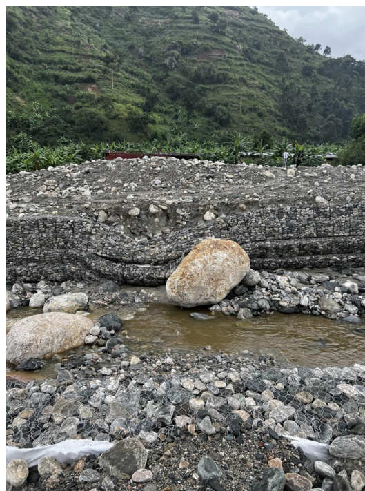
Figure H2. 0.21387° N, 30.00558° E, 7 June 2023 (damaged gabions).
