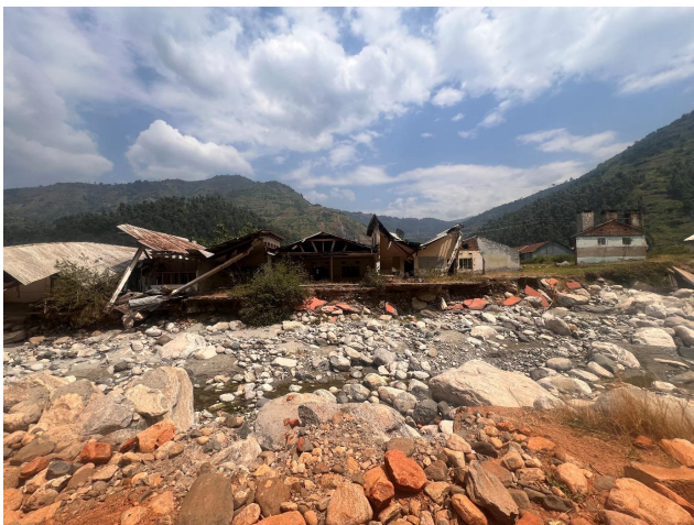
Figure F2. Riverbank style erosion of house foundations in Kilembe, 0.20603° N, 30.00822° E – 24 July 2024.
