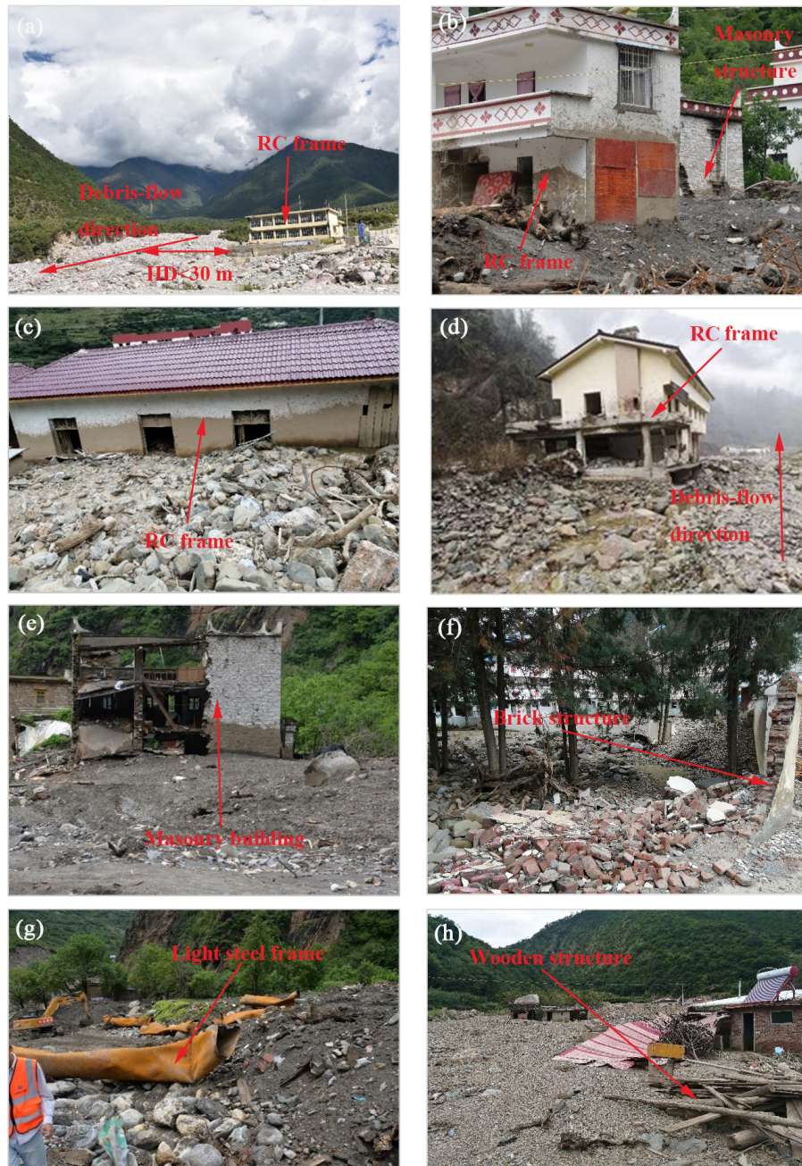
Figure 4. Photographs of the damaged residential buildings caused by debris flows during field investigations on the Qinghai–Tibet Plateau.
