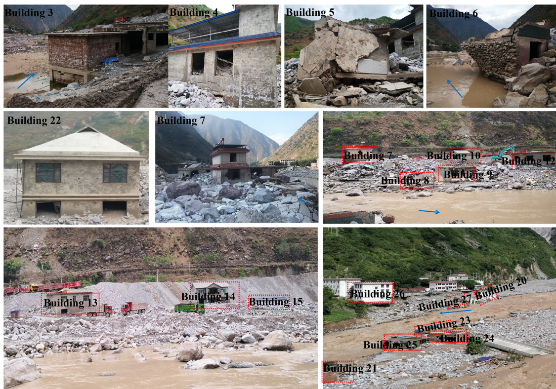
Figure 13. Buildings with different degrees of damage within three hazard zones.
