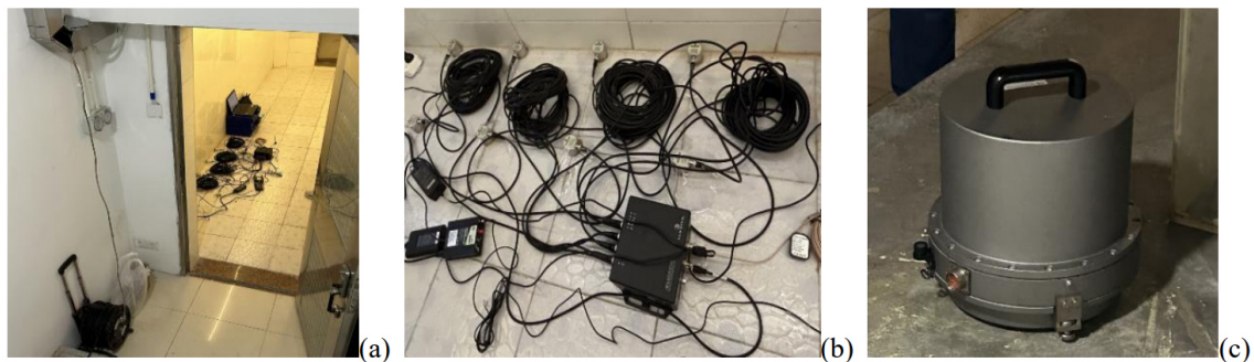
Figure 5. Setup of monitoring system. (a) Interior view of the tunnel, (b) AE acquisition device and (c) seismometer.
