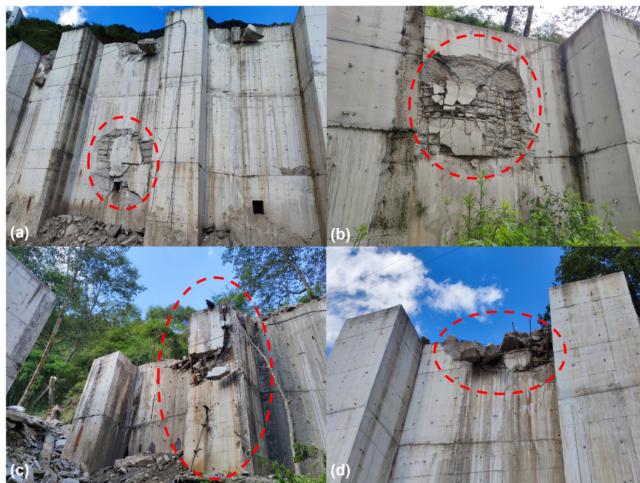
Figure 1. PSRWs in southwestern China in (a) Kongyu, (b) the Jiuzhaigou nature reserve, (c) the Zhenjianguan tunnel exit on the Chengdu–Lanzhou railway, and (d) Zhangmu.
