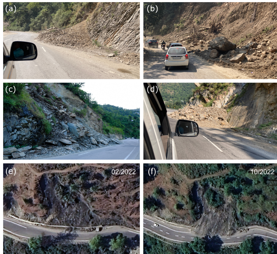
Figure 2. Examples of partially road-blocking landslides along the highway NH-7. Panels (a) and (c) show locations where hillslopes parallel the foliation and/or bedding. Panels (e) and (f) show a landslide that was reactivated in the observation period (Google, © 2024 Airbus).
