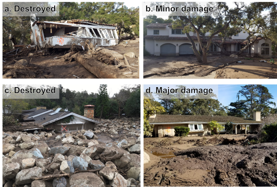
Figure 2. (a, c, d) Examples of buildings that were classified as sustaining major damage or destroyed from different locations in the San Ysidro runout path (locations depicted in Fig. 11). Some buildings had the entire first floor wiped out (a, CAL FIRE building damage ID 437), others were inundated by boulders (c, CAL FIRE ID 268), and others were impacted by mud (d, CAL FIRE ID 100). Panel (b) (CAL FIRE ID 389) depicts a building that had minor damage. All photos from Kean et al. (2019a).
