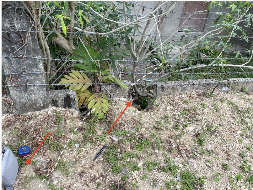
Figure S12: Pt FC22. Fence adjacent to the septic tank showing sinistral offset.
