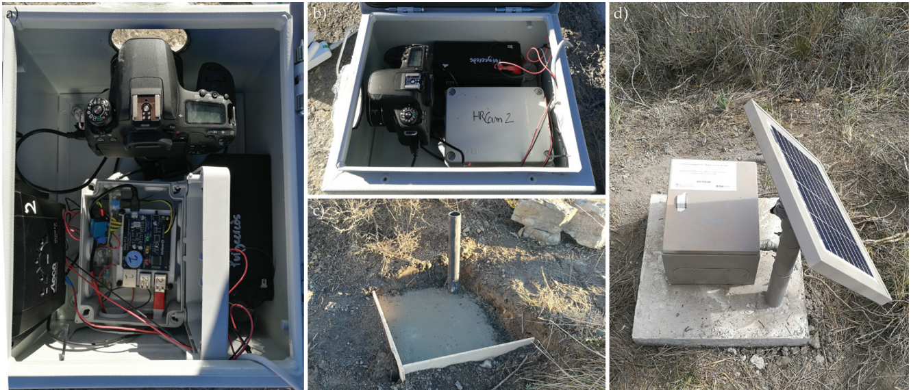
Figure 1. Images of the photogrammetric systems installed in the Puigcercós site: (a, b) Fig. 3 shows the inside of the photogrammetric unit with part of the connections; (c) construction of the concrete base and installation of the PVC pipe for the installation of the photographic units; and (d) external view of the installed system.
