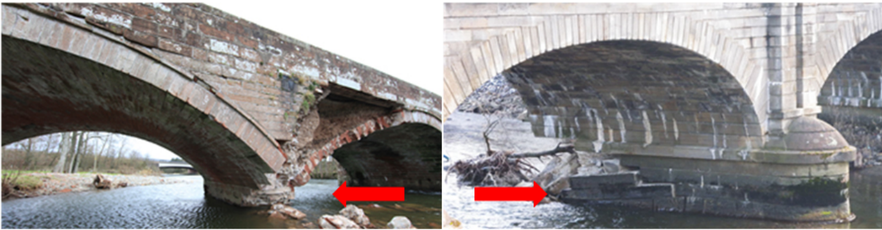
Figure 2. Damage of Brougham Old Bridge (a) and of Calva Bridge (b), typical of many masonry arch bridges subjected to scour (source: Cumbria Council County for a and Bill Harvey for b). Flow direction indicated by arrow.
