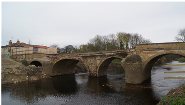
Figure 3. Tadcaster Bridge, damaged by Storm Eva in 2015, repaired and reopened to traffic 13 months after. Bridge closure resulted in a 9 mi (14.5 km) detour of 20 min to reach the other side. Source: https://commons.wikimedia.org/wiki/File:Tadcaster_Bridge_closed_following_last_years_damage_(10th_April_2016)_005.JPG (last access: 3 March 2022).
