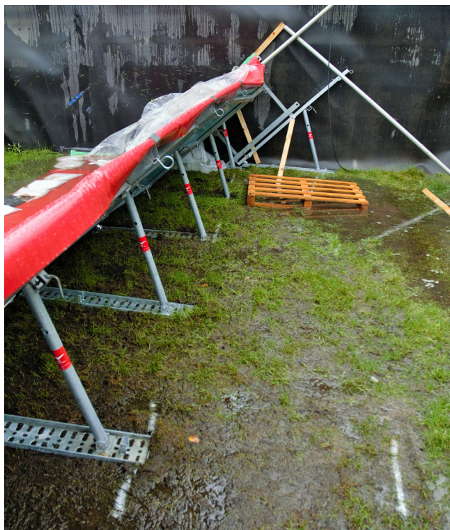
Figure 10. Supporting columns sunk into the saturated foundation soil after damming (aqua defence).
