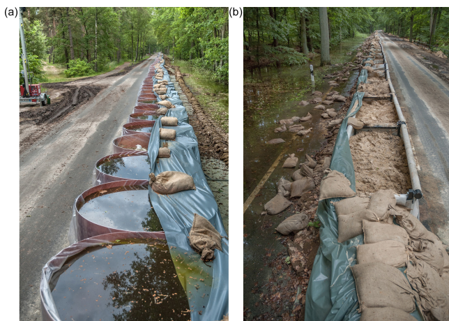
Figure 4. SBRs near Gartow (Lower Saxony, Germany) after the Elbe flood in 2013 using (a) AQUARIWA and (b) Quick Damm Type E.
