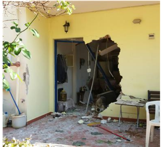
Figure 3. Damage from the falling rock on the impacted house in Ponti, Lefkada, Greece.
