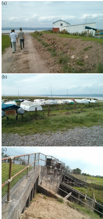
Figure 4. (a) Thornbury Sailing Club: Localised club sea defences can be seen to the right of the track (Note: This area is situated between High Water and EA sea defences). (b) Thornbury Sailing Club: Adaption to flooding events (boats stored on stilts) (Note: This area is situated between High Water and EA sea defences). (c) Oldbury Pill flood gate: One of the lower points indicated by LiDAR. Debris can be seen in the foreground indicating the likely water level of the January 2014 event.
