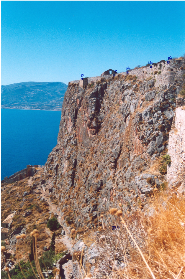
Fig. 2. Photo of a section of the high rock slope and the Monemvasia historical site (Section C in Fig. 11).
