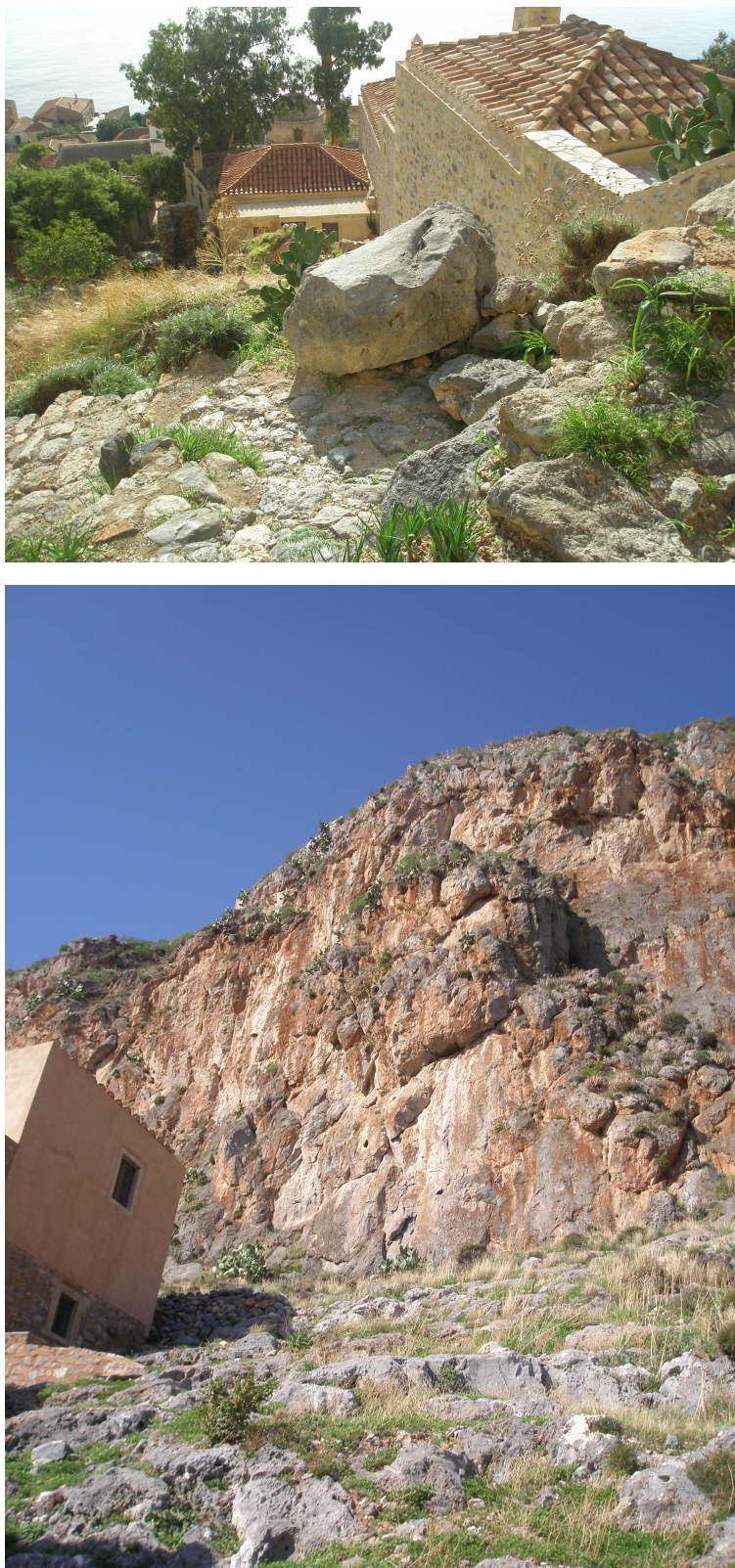
Fig. 3. (a) View of fallen rock blocks in area of section D (b) overhanging blocks in area of section Z. Range of volumes: 1.5 to 5 m 3 .
