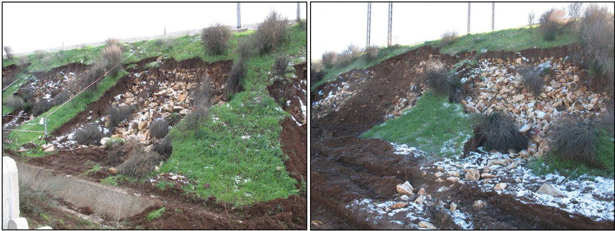
Fig. 14. Unravelling/sliding failures observed along the slopes of the remaining portion of the Acquaviva embankment.
