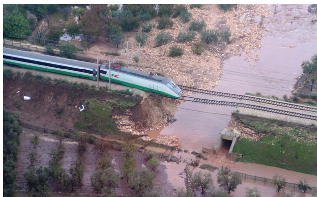
Fig. 3. View of the breach developed in the Acquaviva railway embankment (point 4 in Fig. 4) after 5 October 2005 flooding (picture taken from the upstream side).
