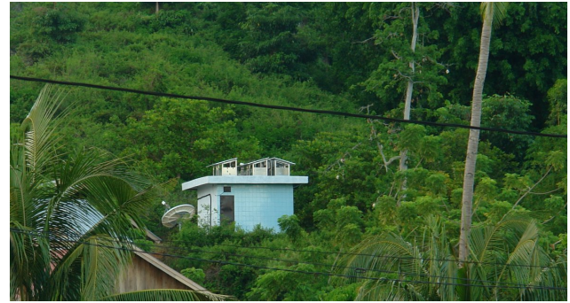
Fig. 17. Remote seismic sensor station with solar panels for the power supply of the sensors, the processing system and the communication link (Sanana, Moluccas Islands).
