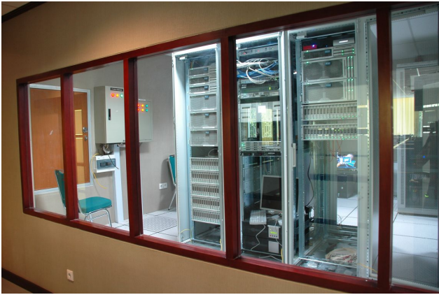
Fig. 16. Local infrastructure in the warning center in Jakarta for the processing systems in the server room.
